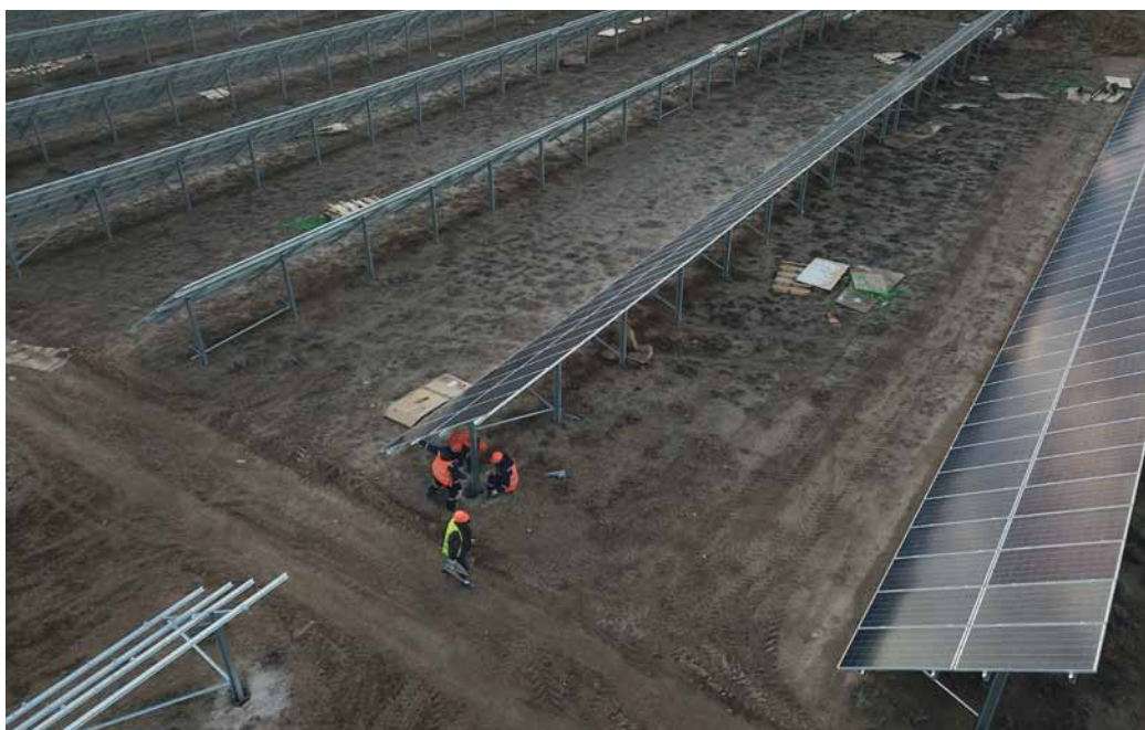
This 50 MW solar PV power plant, and its subsequent 26 MW extension array, are located in the Karaganda region, in central Kazakhstan.
